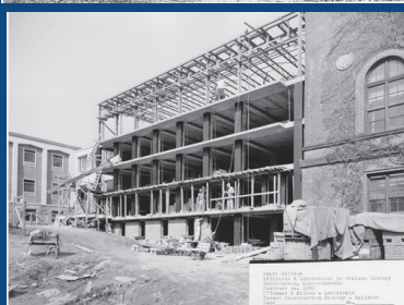
Demolition of North Wing's Little Chapel location to make way for Northwest wing. Construction of the Northwest facade of Neilson 1961 and Completed Northwest wing facade, 1962.
