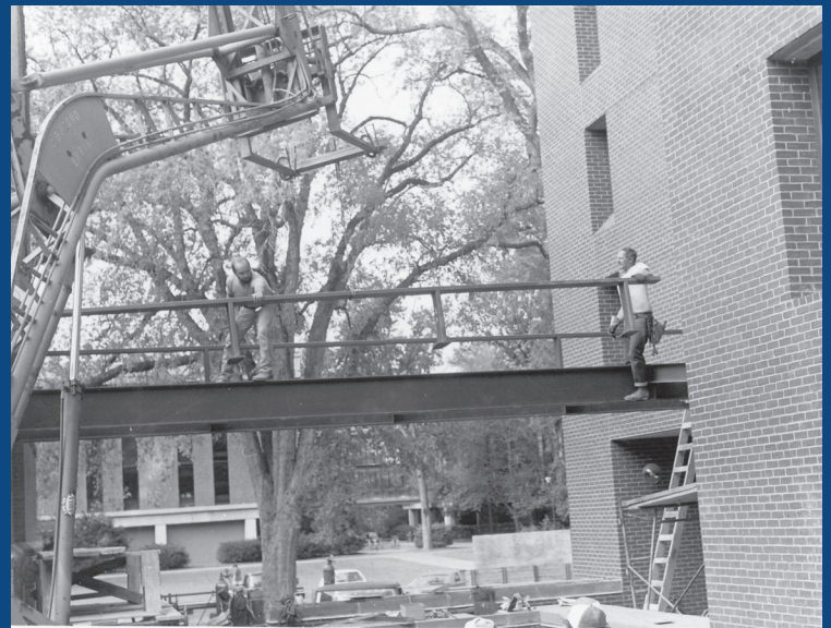
Installation of steel beams for glass connector between South Wing of Neilson and Alumnae Gymnasium, ca. 1980.
